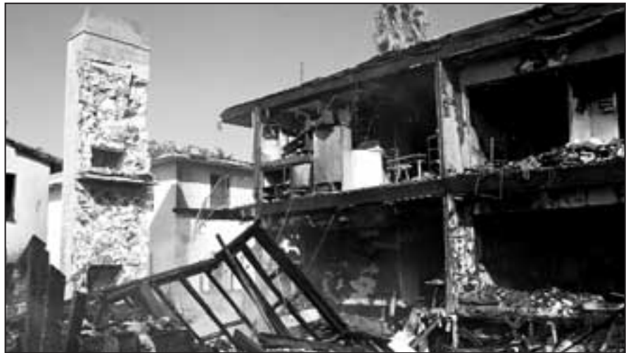
Partially collapsed building due to fire damage.
